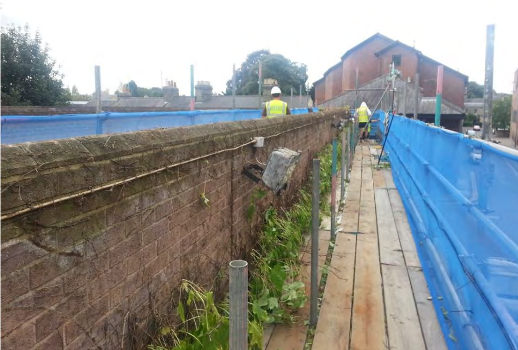
General Views of the unstable access ramp wall
