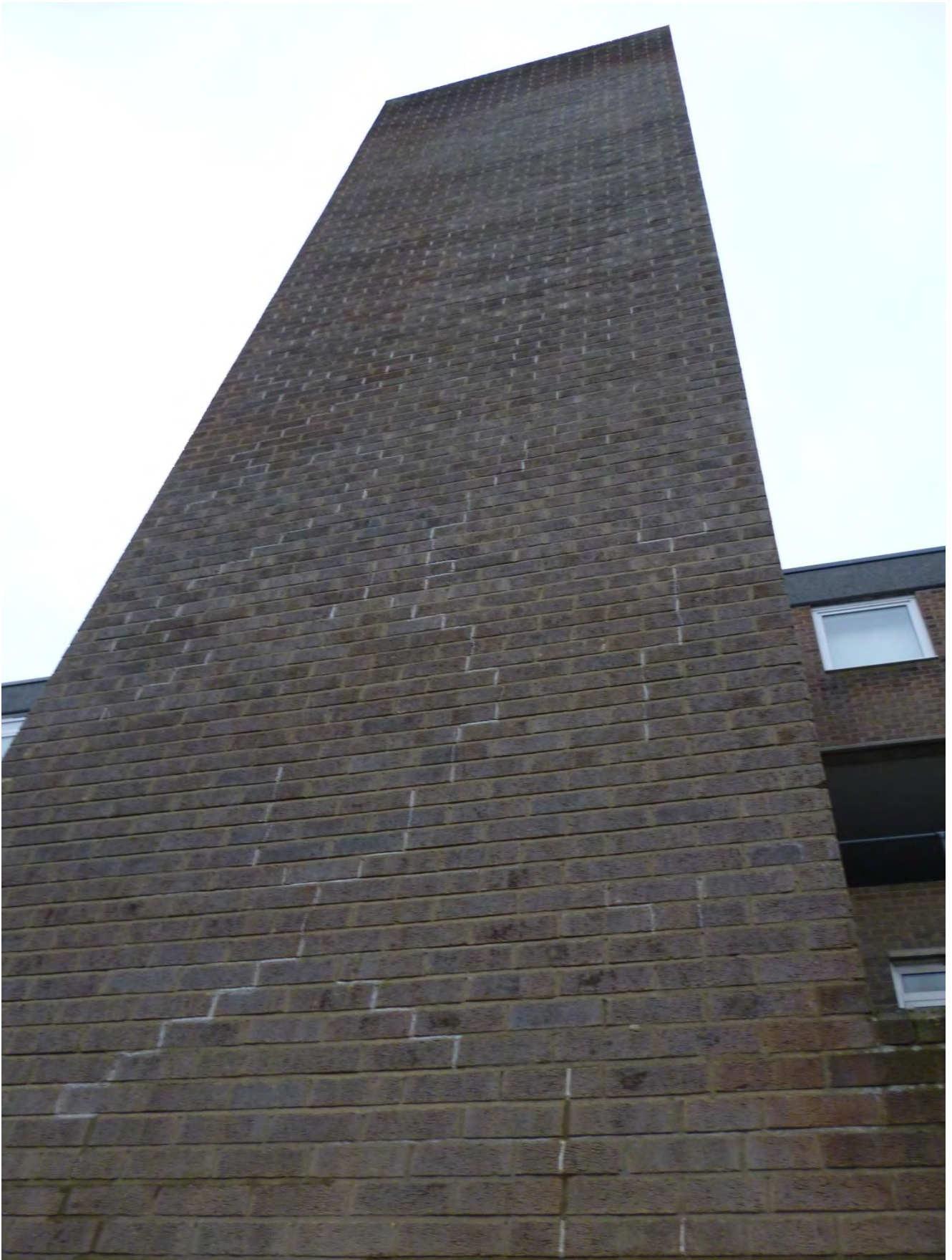
Example of - Crack Tracing on Princess Bin Chute Tower prior to Year 2 repairs
