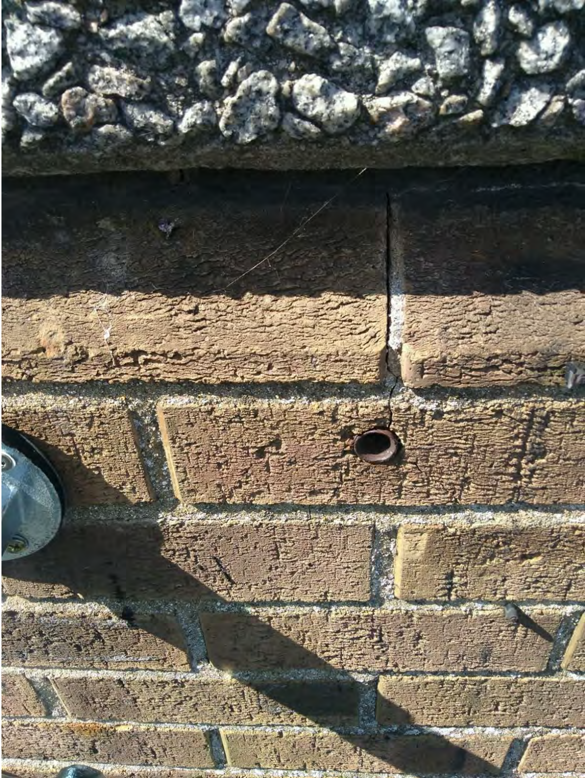
Typical Examples of Old Fixings left Rusting and Expanding within the Masonry Façade of the Buildings
