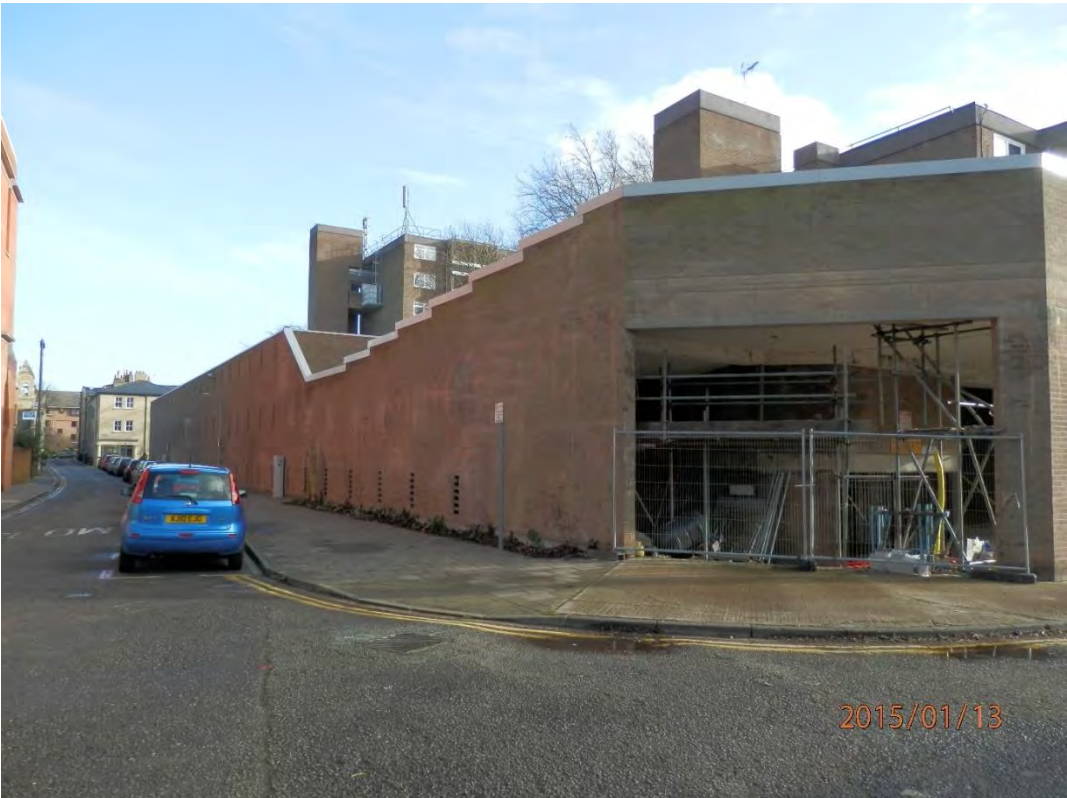
External View - after the Year 0 Remedial works and the reduced and tied back external wall located aside the car access ramp.
