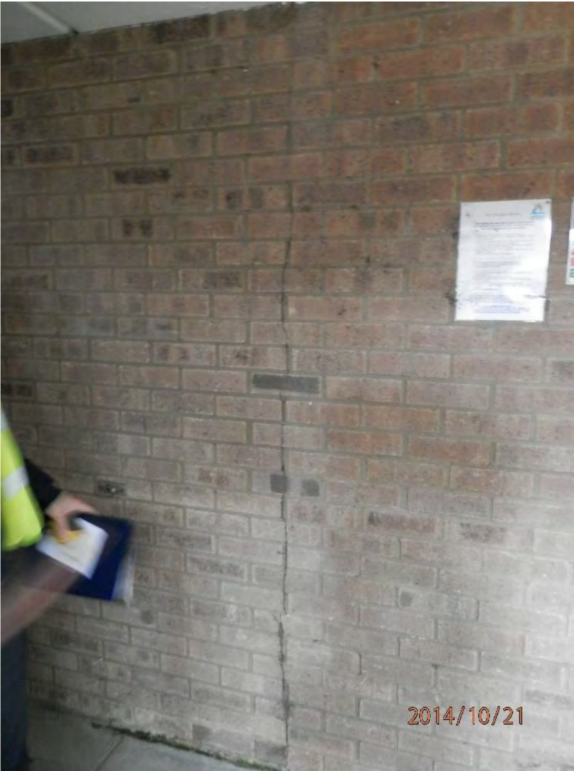
Eastern Staircase of Hanover Court Typical Entrance Structure - Cracking Internal Northern Side: Repaired in Year 1 Urgent Works
