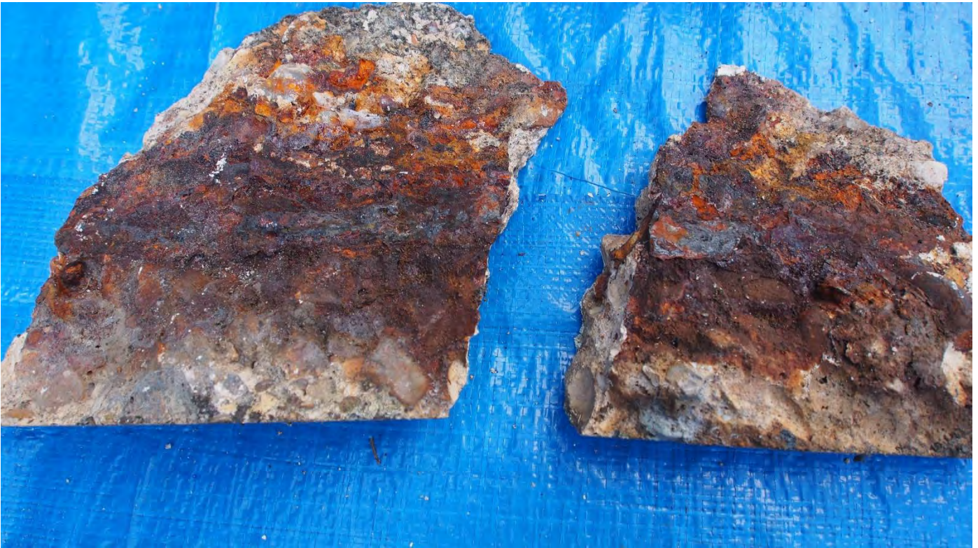
Typical Removed Section of Balcony Panel Bottom Drip Detail found loose and painted over Loosened due to steel bar corrosion
