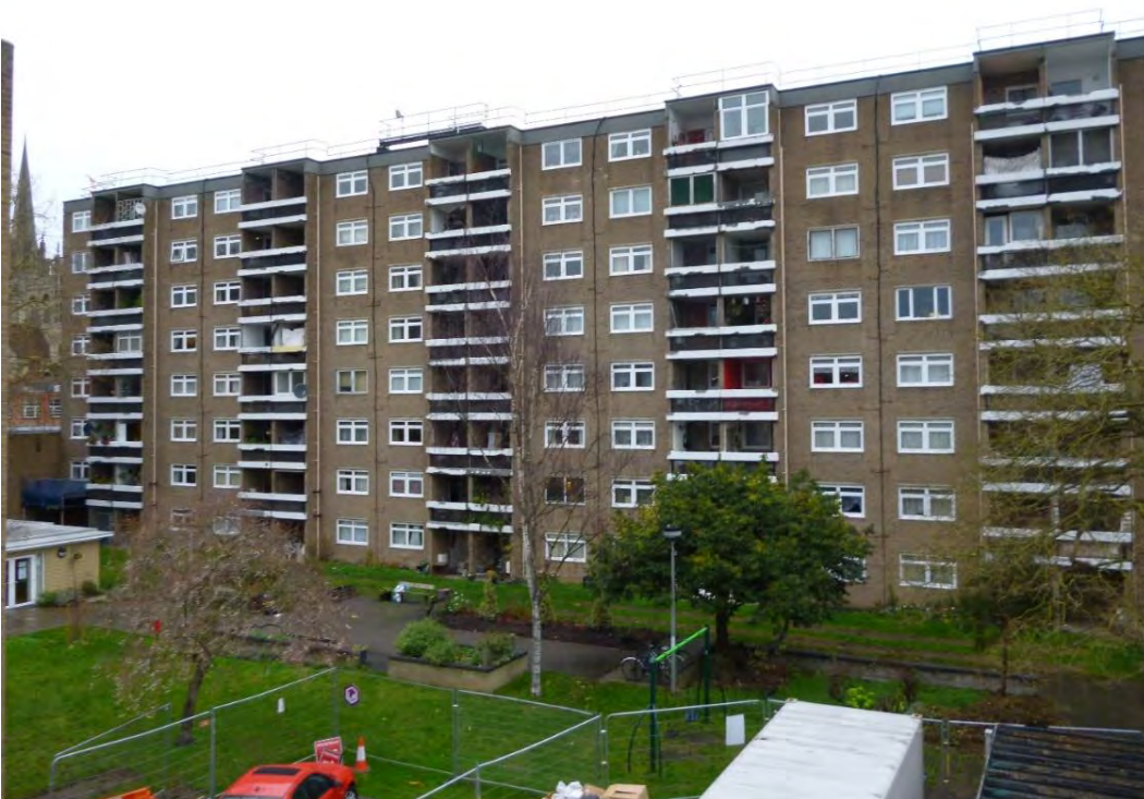
Hanover Court Western Elevation: - Note the grey Sika 903 and Sika 610 temporary blinded areas on the concrete balcony panels. See SJW Photographs and lists of the defects and locations and MLTS Ltd Drawings for overall view of these records.
