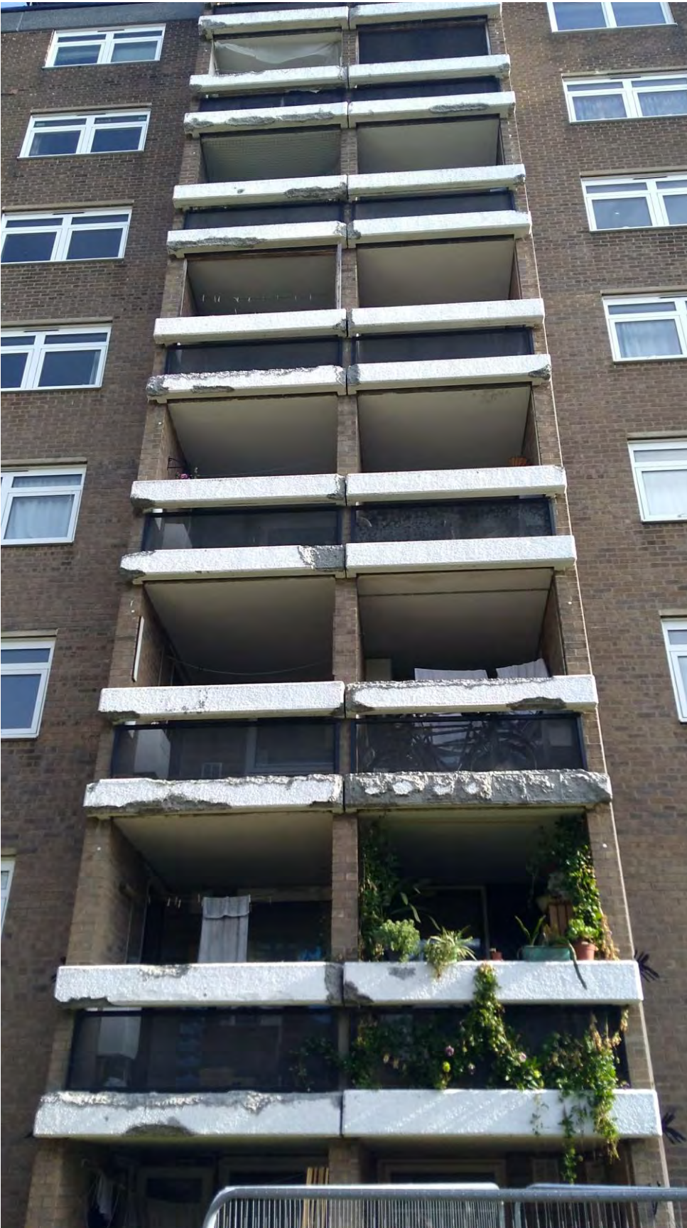
Hanover Court Tap Tested and Primed Panels with SIKA 903 and SIKA 610 Locally – Typical Example
