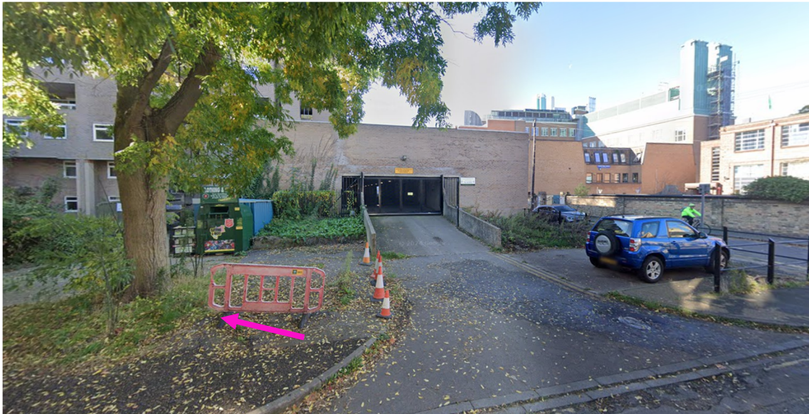
Image 4 – The existing hard surfacing will be used for the Construction Site Offices and Pedestrian Turnstile. G003 is on the left side of the image. Temporary protective fencing to be installed at the kerb edges.
