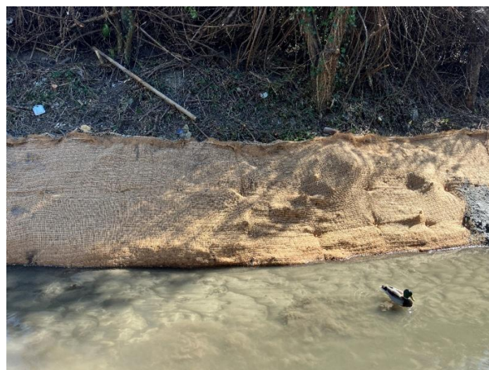
Coir matting to stabilise eroding banks and establish native marginal plants along Cherry Hinton Brook
