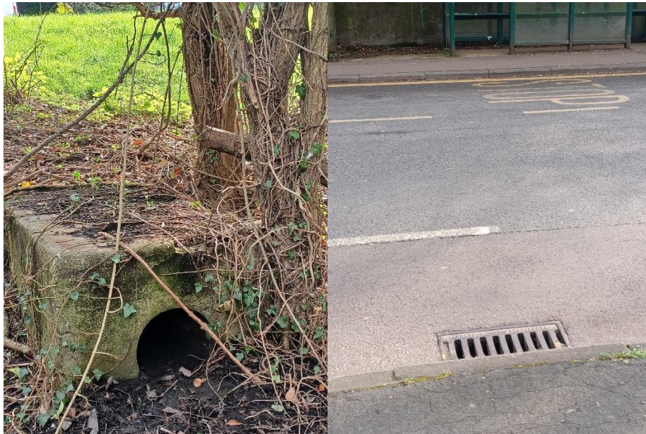
Highways drain and outfall pipe discharging urban pollution into Giant's Grave
