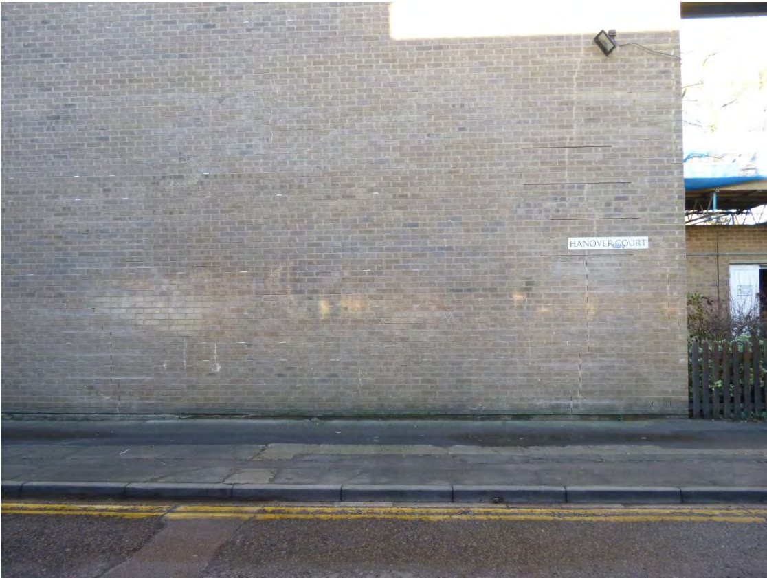
Hanover Court Sample Gable End Panel Tracing Brickwork Ties – Note the unusual pattern
