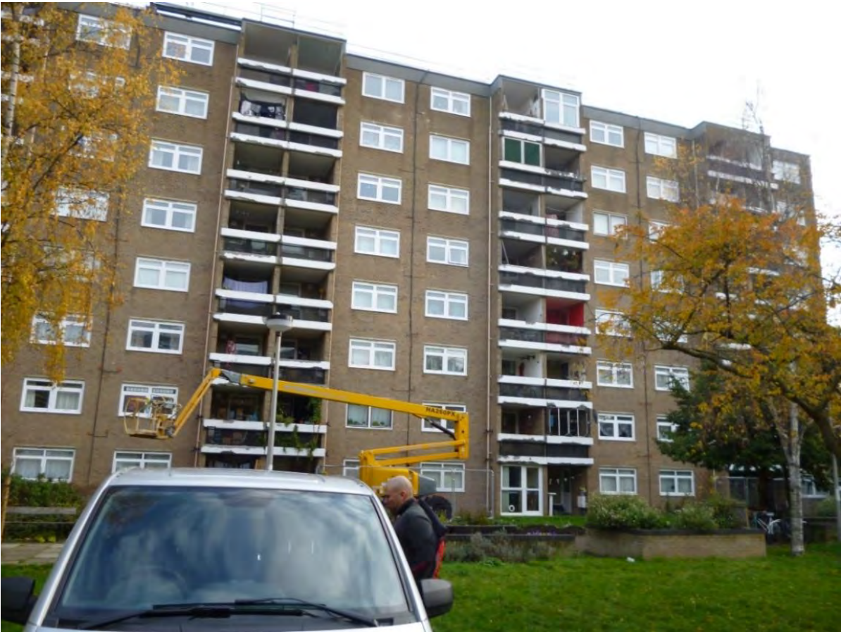
Hanover Western Side - Note the mobile access platform used to access and repair Hanover Court Building initially the Parapet panel Repairs and then the Balcony panels Tap Testing to remove loose concrete. .
