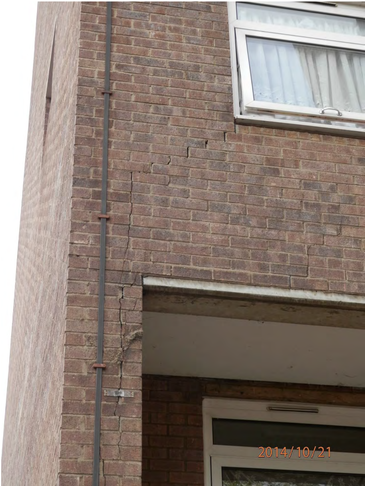
Year 1 and 2 Emergency Repairs due to wind loading acting with dead and live loading
