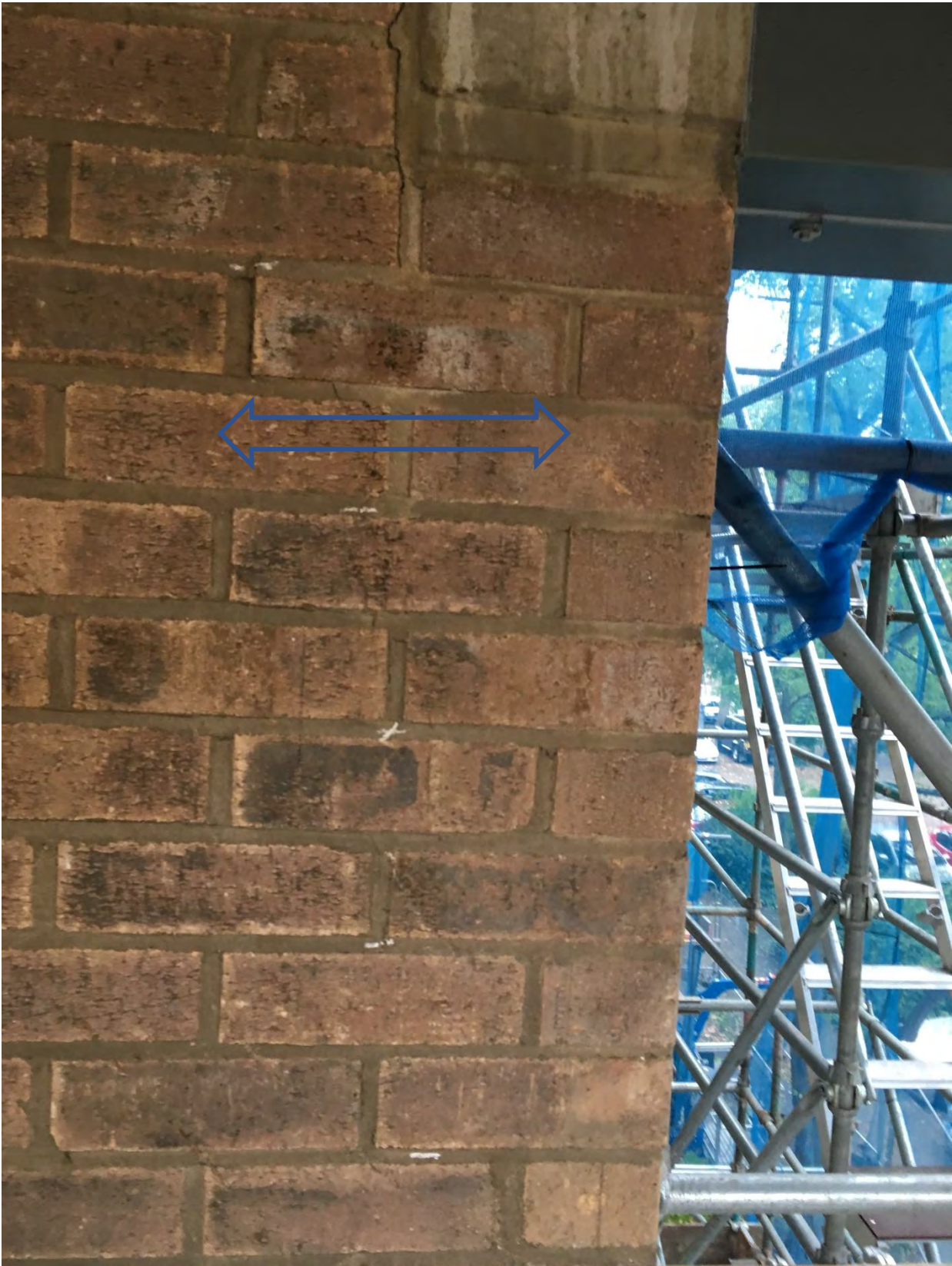
Cracked Walkway Beam Bearing onto the Hanover Court Building – Note the tracing of the brickwork ties
