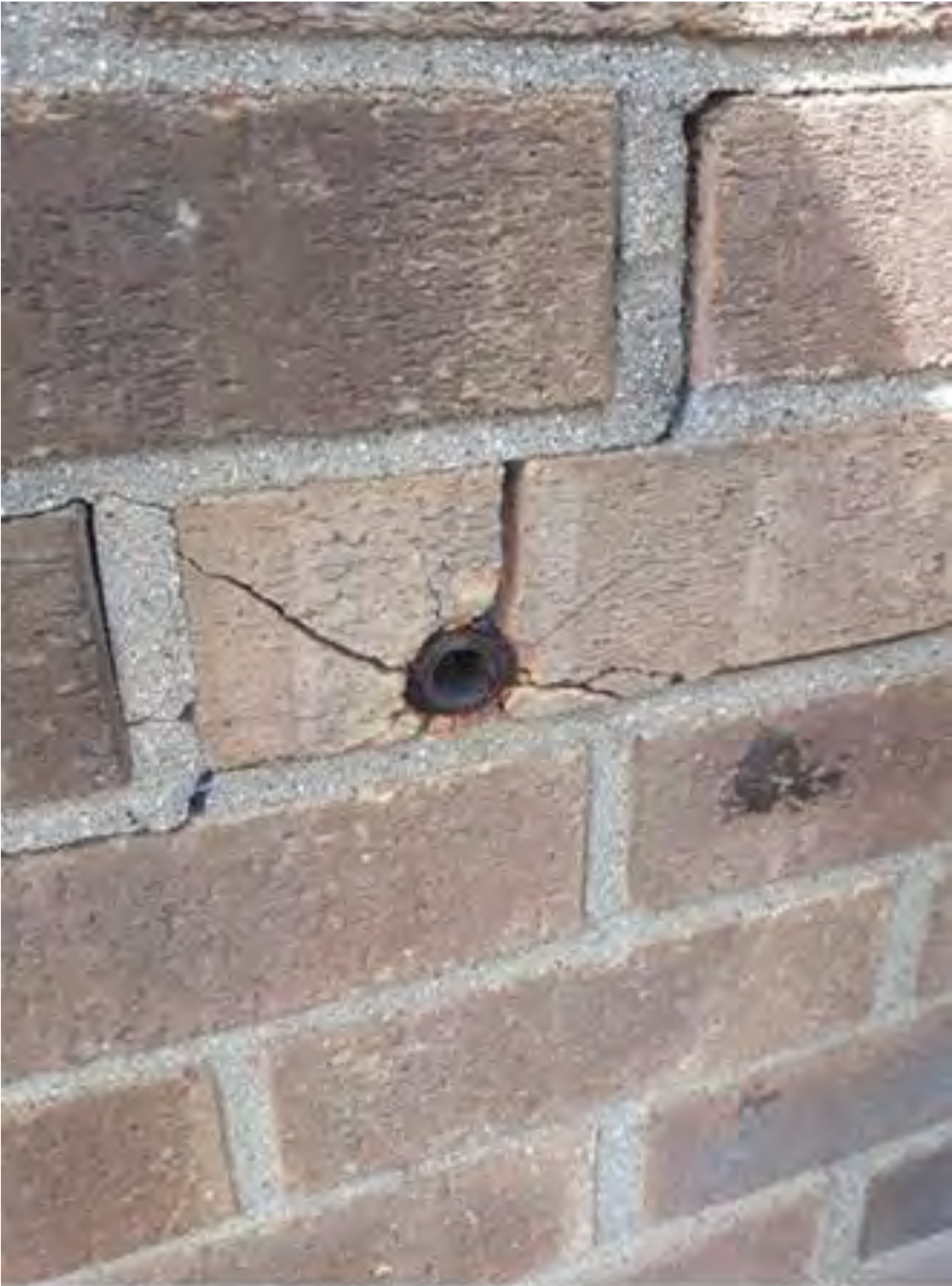
Top of Princess Court Bin Chute Tower corroded old Scaffold Fixing bursting the brickwork at High level
