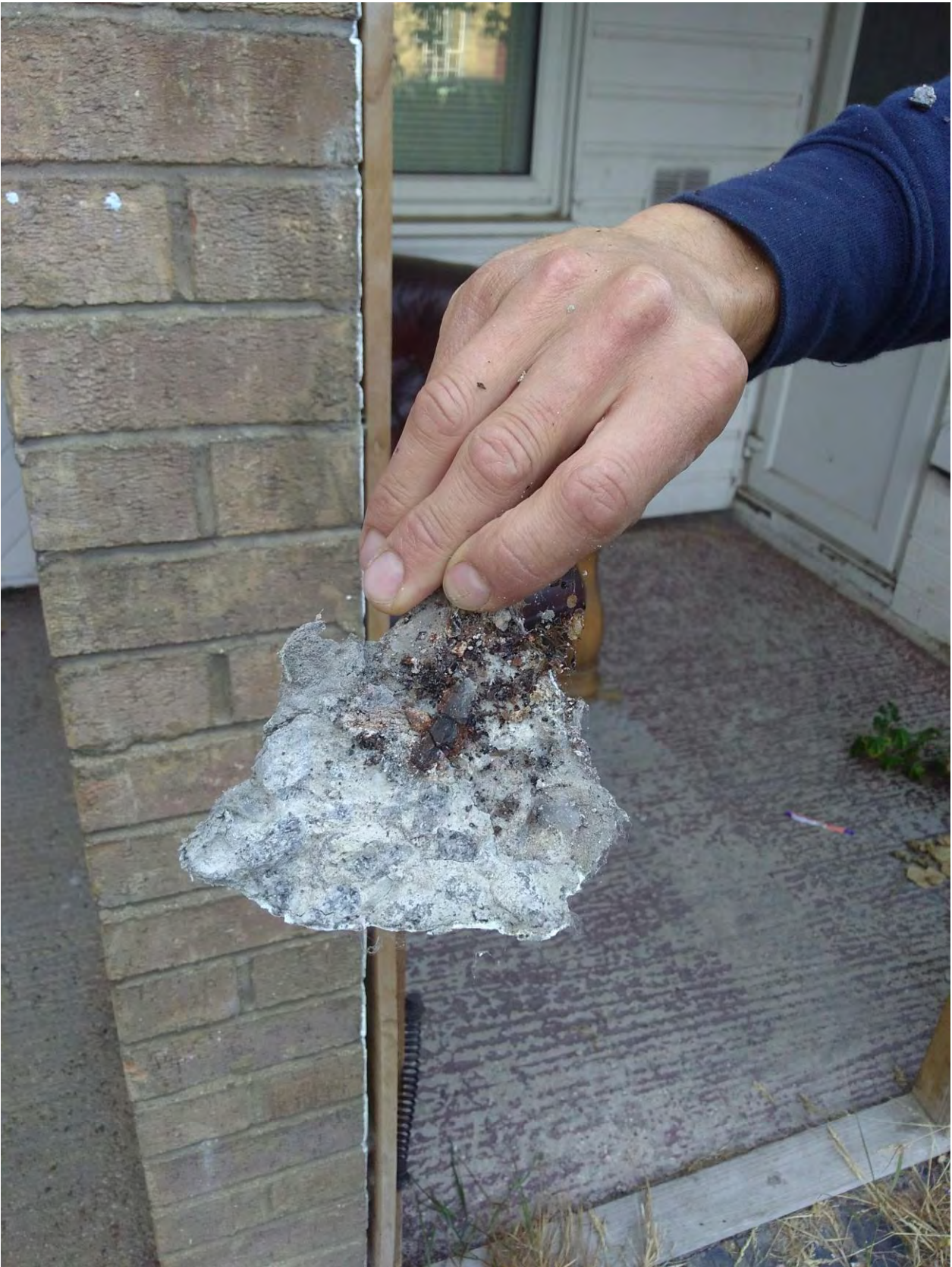
Typical loose Balcony panel corner Removed Easily by Hand.
