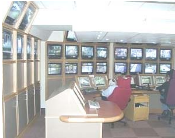
CCTV Control Room
