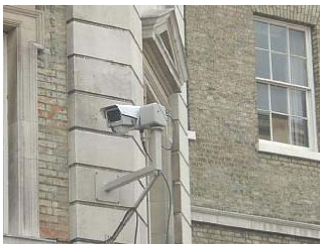
Wall Mounted Fixed Location CCTV Camera
