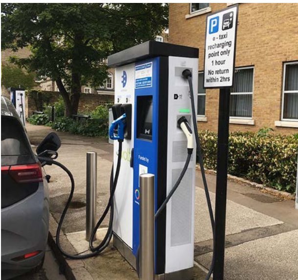
Electric taxi recharging point
