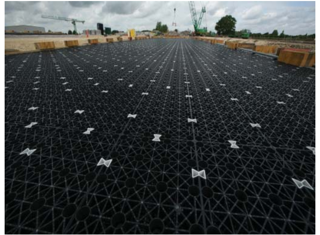
Shallow geocellular storage used below permeable paving as a subbase replacement at a Park and Ride site in Cambridgeshire
